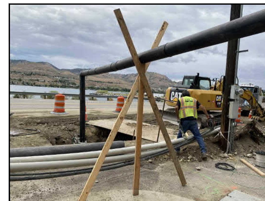
TEMPORARY FORCEMAIN BYPASS
